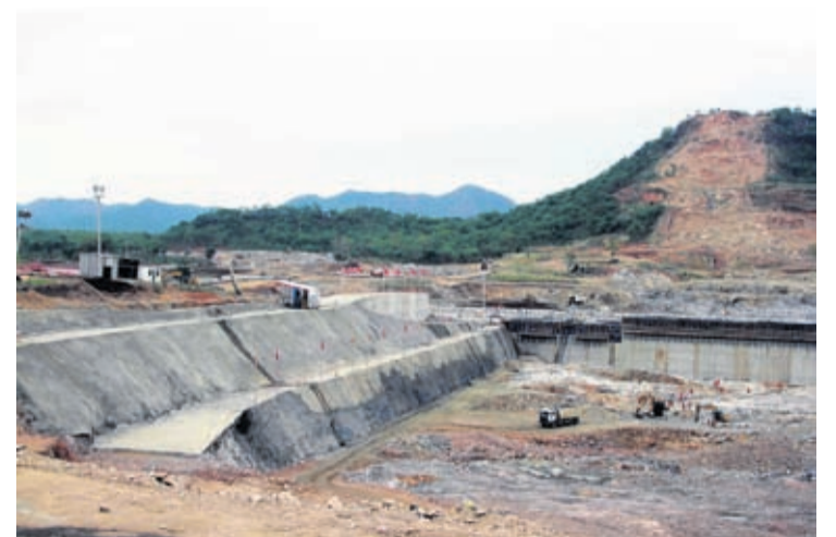
BANDA In this June 28, 2013 file photo, construction work takes place, at the site of the Grand Ethiopian Renaissance Dam near Assosa, Ethiopia.
